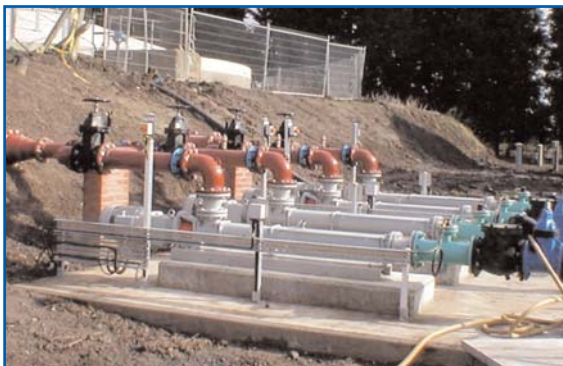
Duty/standby pumps circulating sludge with a high rag content from digesters
