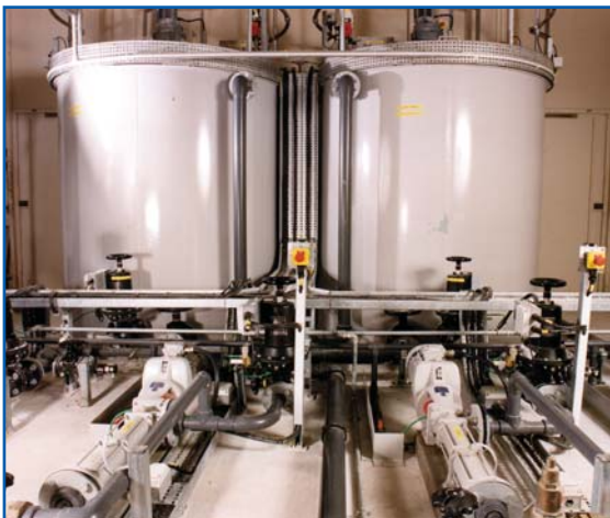
Accurate controlled pumping of hydrated lime solution from slurry mixing tanks to the dosing points
