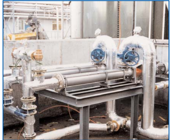
Slurry mix at this paper mill is pumped in a recirculation loop to a dosing valve and back to a holding tank
