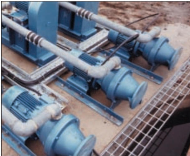
M18 Macerators, part of a Mutrator system installed to macerate settled sludge and storm tank effluent.
