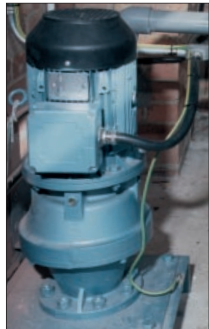
M180 mm Vertical Macerator installed as part of a pumping system to handle sewage from a primary school.
